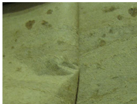
Figure 9. Structural failure, IP-84
